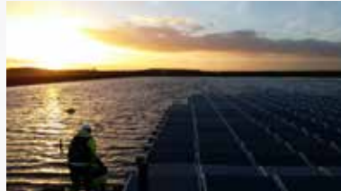
POLYBELL, UK - 471 kWp
