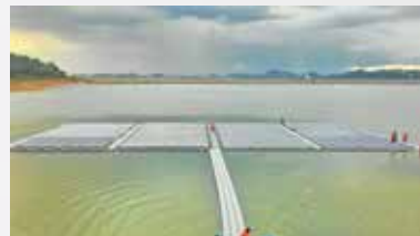
SUNGAI LABU, MALAYSIA - 108 kWp
